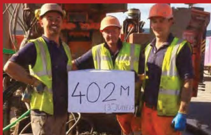
A UK record for the number of metres drilled with one rig in a single day – 2 x 200m double loops installed
