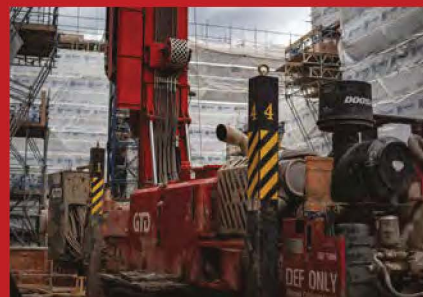
Drilling 50 boreholes to 200m in London saw 1,000m completed in one week
